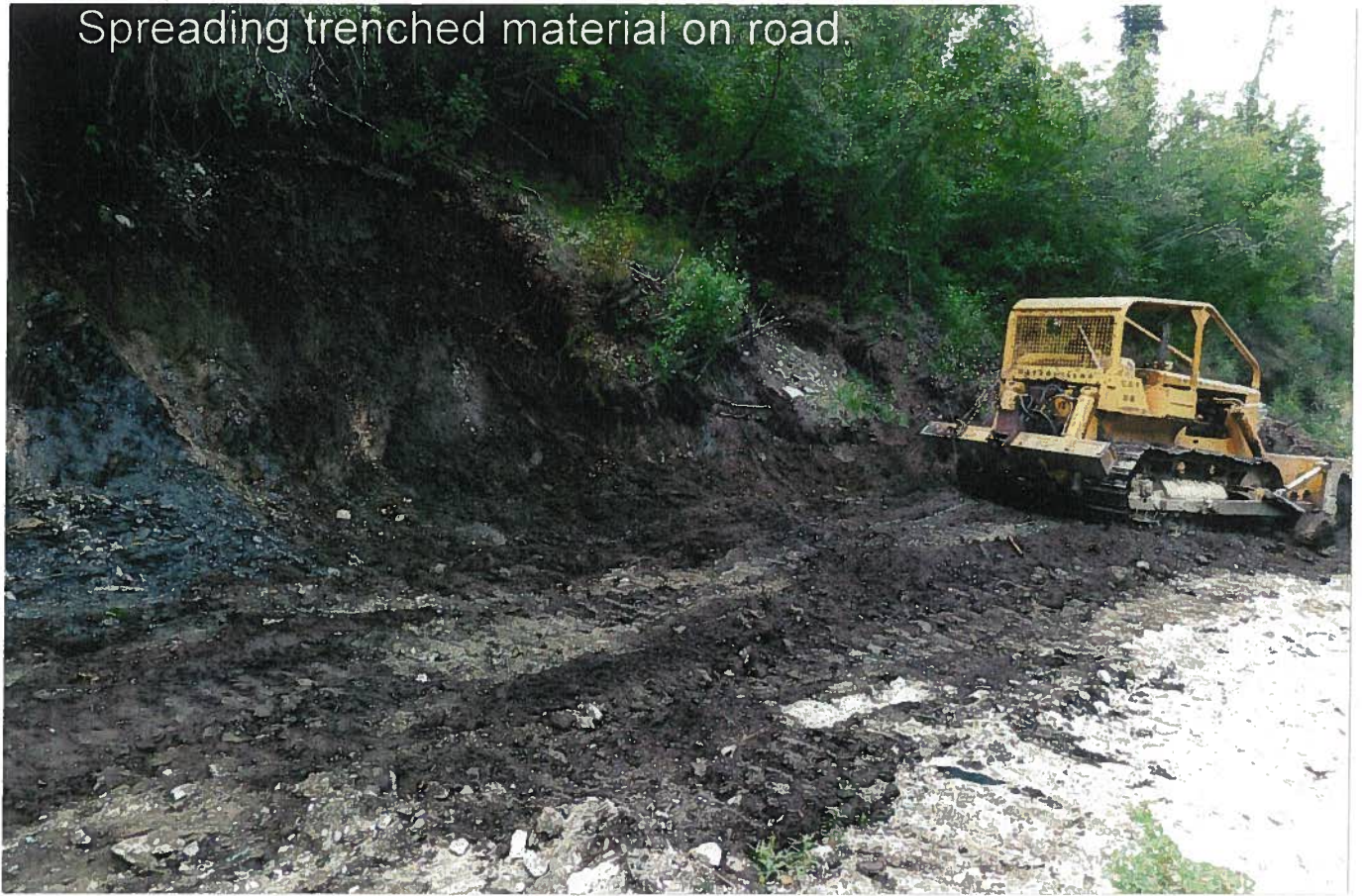
Photo 6: Bulldozer spreading trenched material on road near north end of 2016 Left Limit trench
