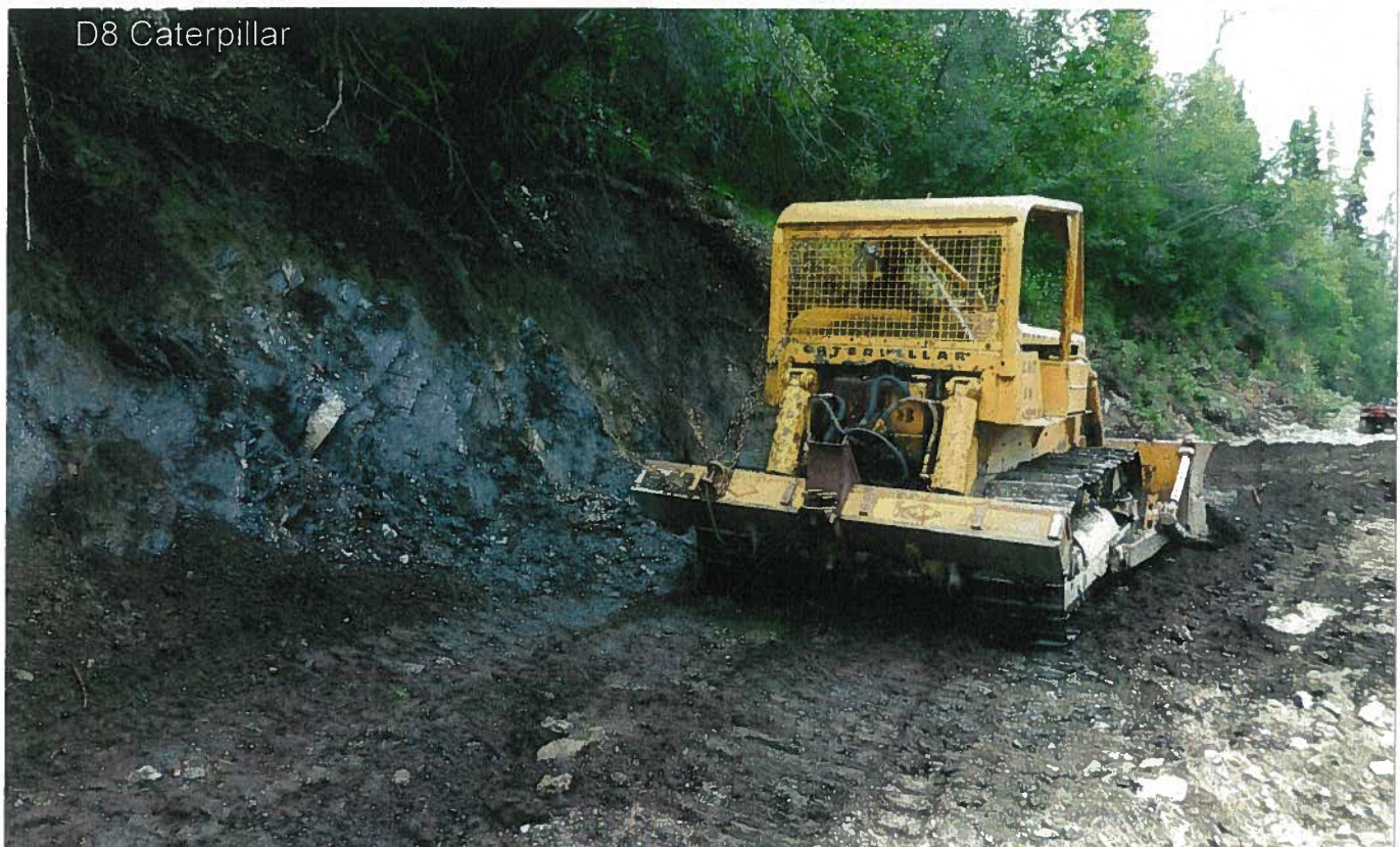
Photo 5: Bulldozer exposing bedrock-gravel contact. Note how high the bedrock is as it rises rapidly to the west marking the edge of any placer gold reserves.
