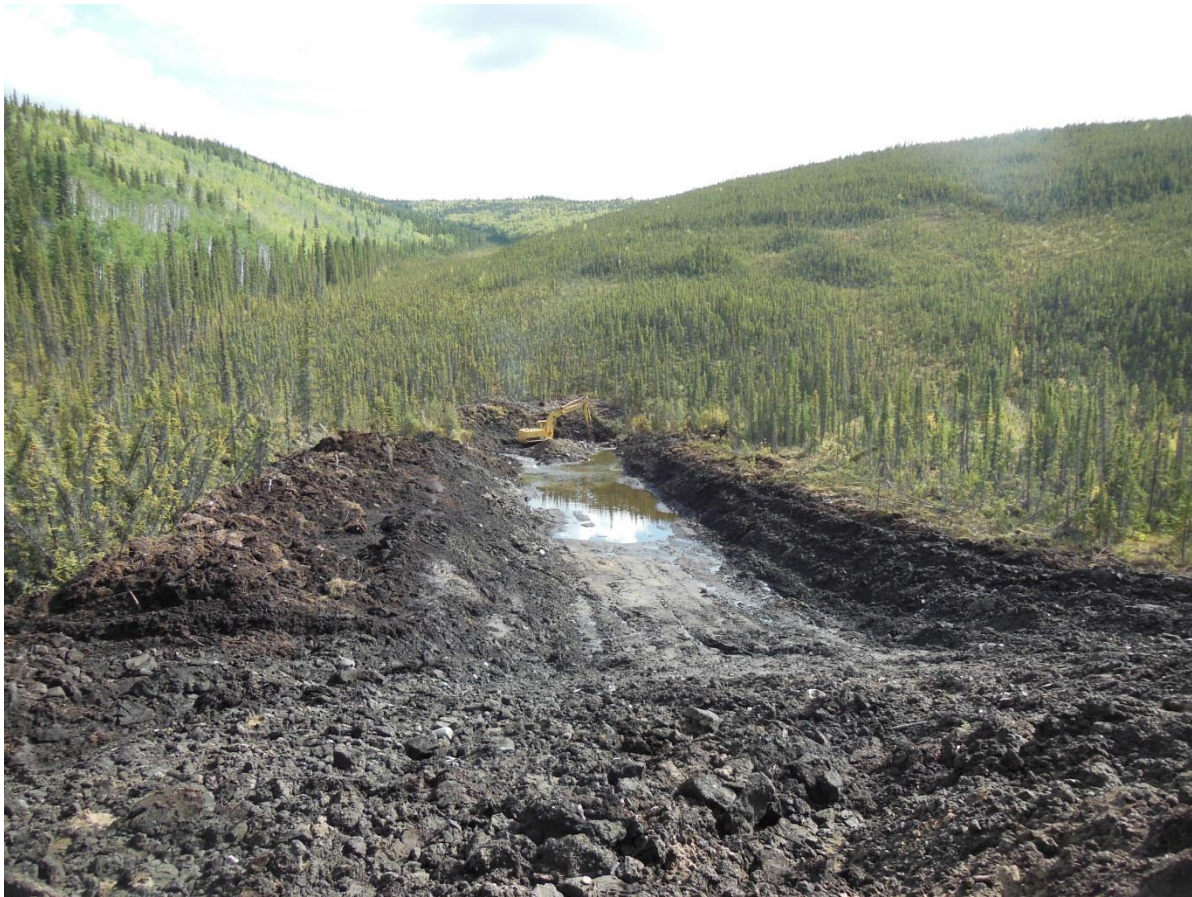
Plate 6 - A view looking south along the bulldozer trench excavated by the D10N. The Caterpillar 225 excavator can be seen at the south end of the trench.
