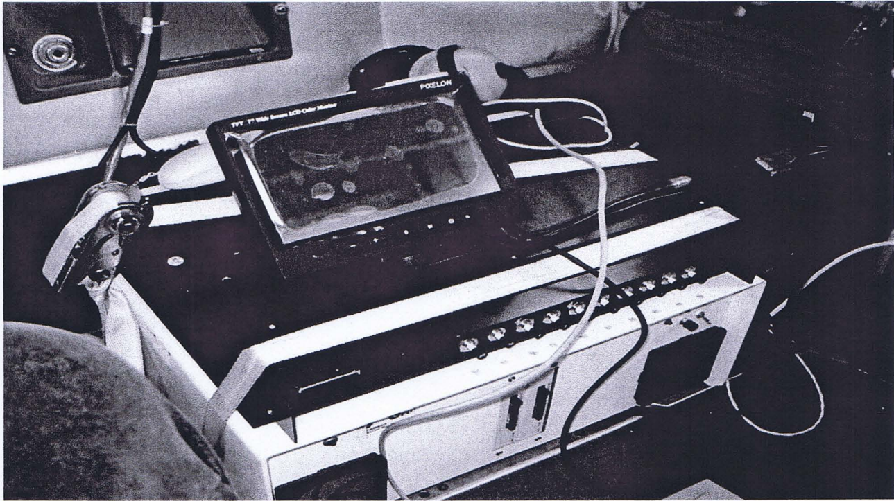
Figure 13: Fluxgeo Data Acquisition System installed in C-GPVN (2006)
