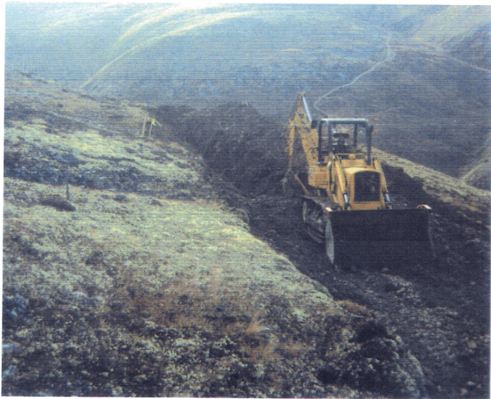
Figure 8. (a) Road construction to Sunrise adit (next to CAT) (b) Trenching T94-1.
