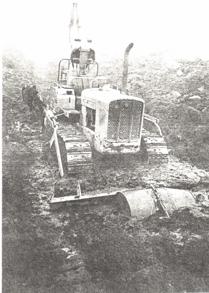
Typical conditions in thawed permafrost.
