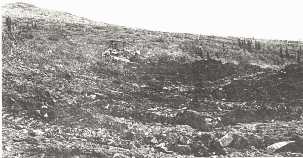
Bulldozers stripping prior to backhoe trenching (removal of vegetation facilitates thawing of permafrost).
