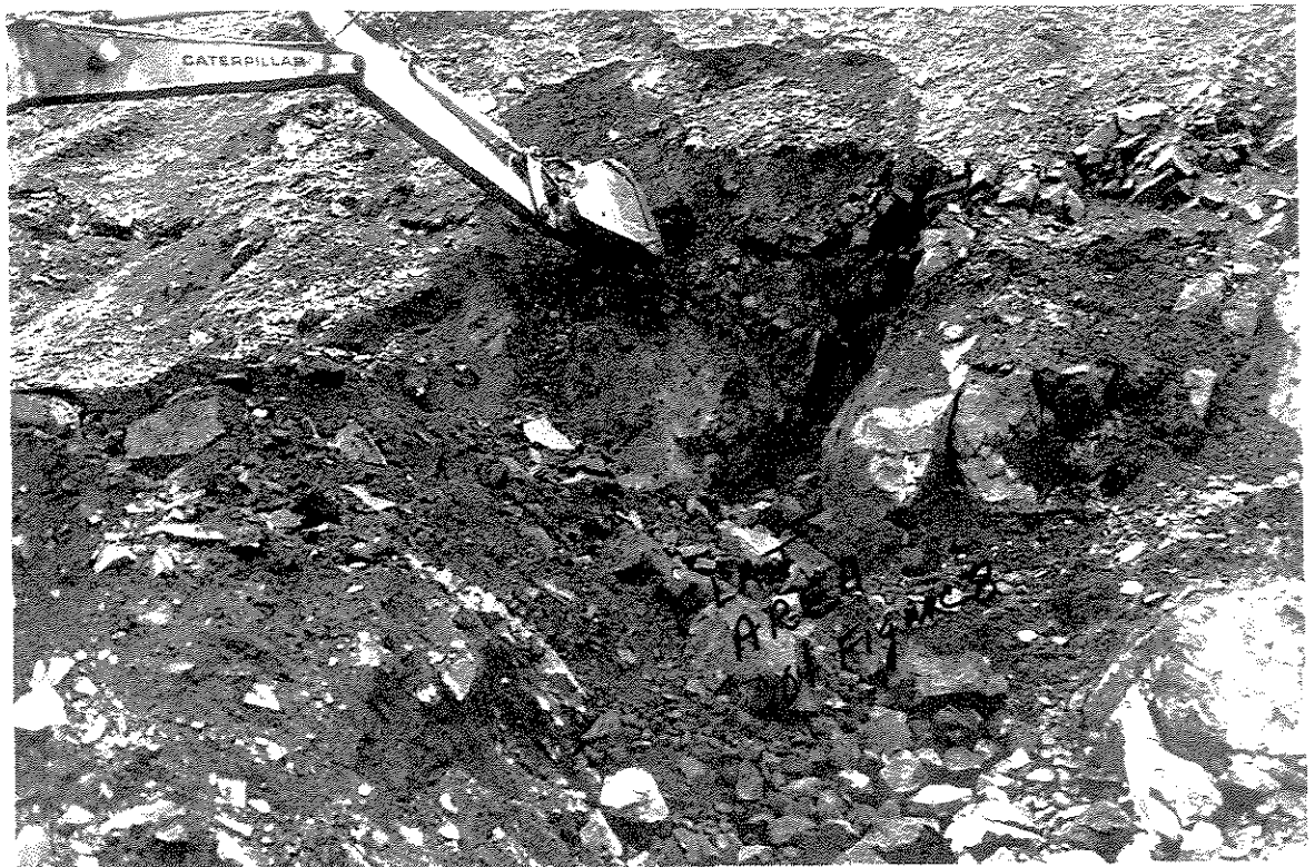
Trenching to the west of high grade zone - needs to be drilled + broken out.
