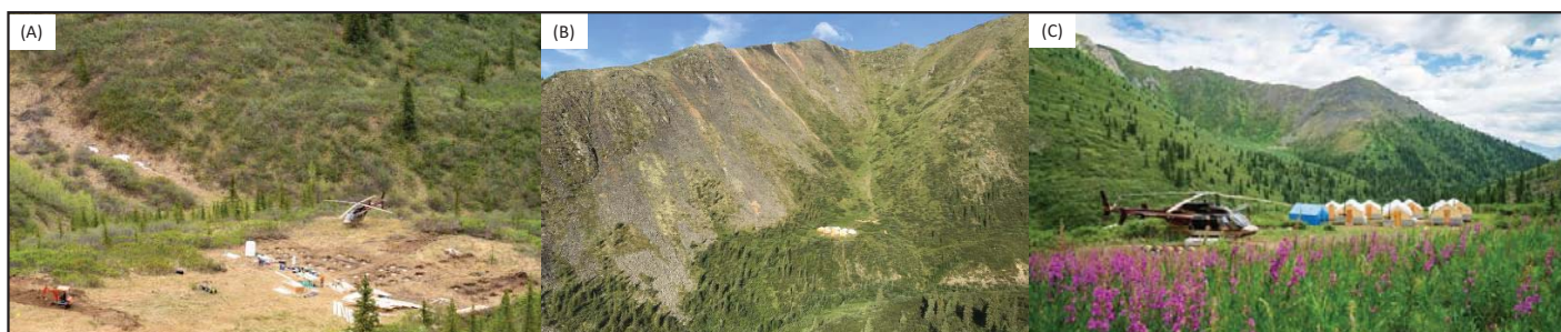
Photo-plate 4. (A) KH41 Heli-portable Kubota working on heli-pad above camp, pads for temporary framed structures being laid out; (B) The new camp was constructed on the north-side of the Central Zone, note Falls Creek in foreground; (C) Completed McKay Hill camp with Bell 407 helicopter in foreground.
