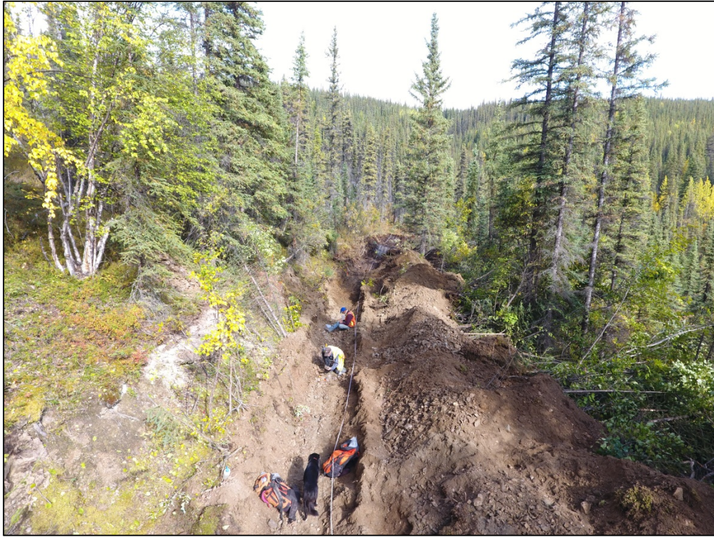
Figure 6. East end of Tr17-2, looking east, note cut bank on left from pre-existing bulldozer Trench.
